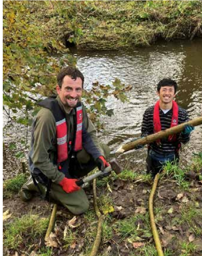
APEM Group's engineers Mike Redding and Vincent Ly used their Volunteer Leave to soft-engineer new river embankments.
